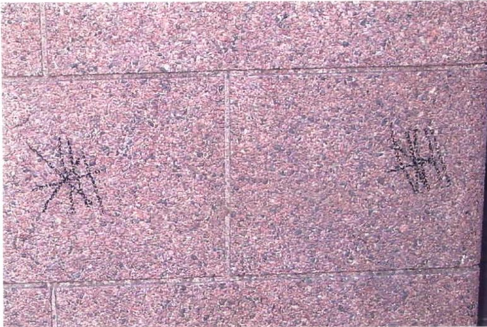
15. Surface with applied graffiti
