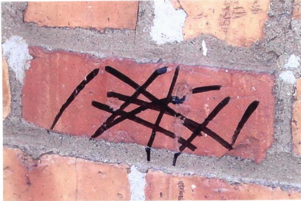
23. Surface with applied graffiti.
