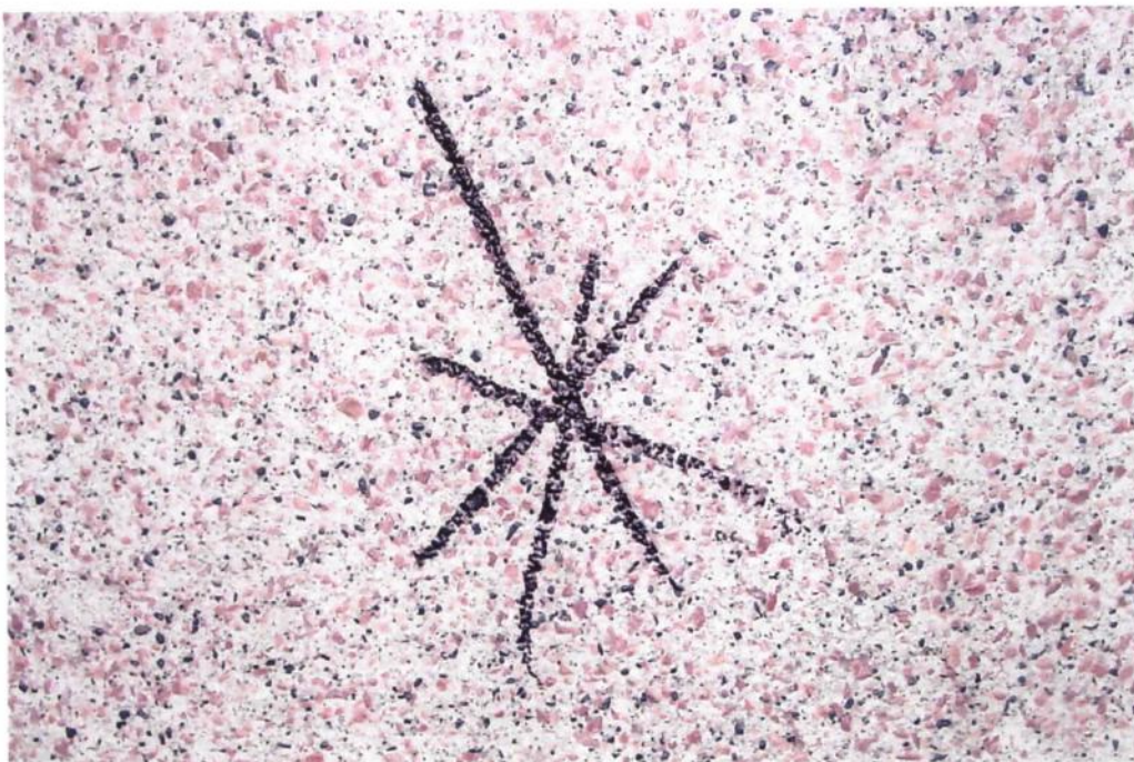
20. Surface with applied graffiti.
