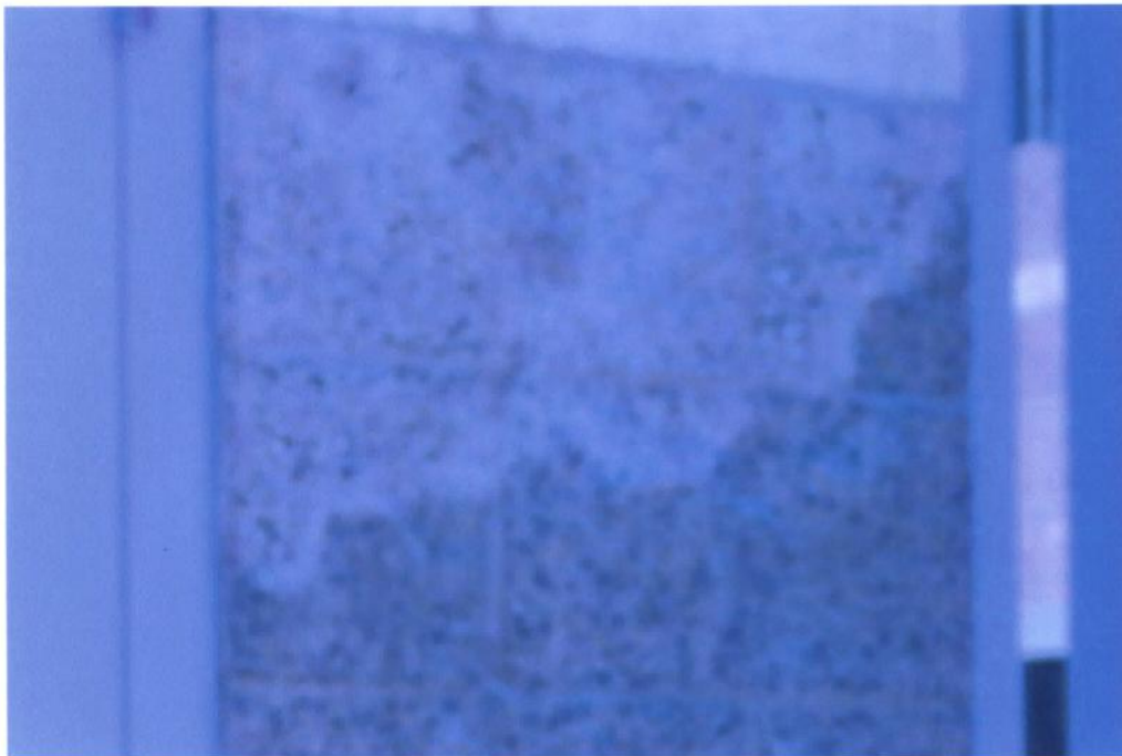
6. View of a wall that was partially sandblasted removing a portion of the GSS system. Note how water intrusion of the unprotected (upper area) has resulted in mottling effect while the protected area remains uniform in appearance.
