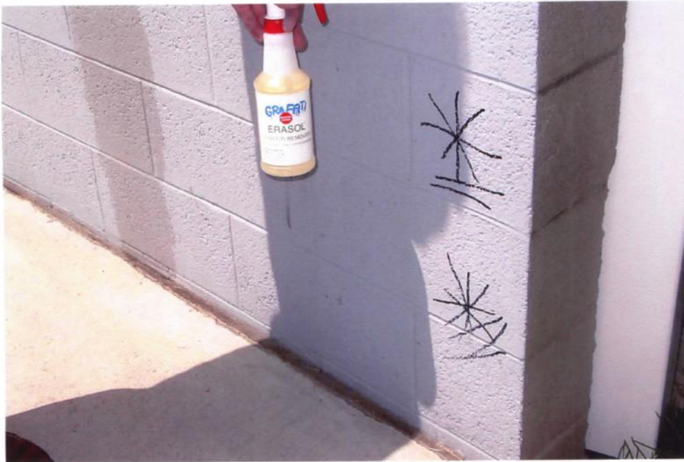
7. Color coated gray, flat GSS system applied to CMU block at the Sandy City Fire Station perimeter wall with black permanent marker type graffiti on the lower blocks.
