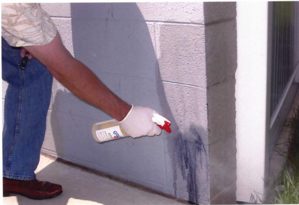
8. View of spray application of Erasol to the graffiti. Note how the graffiti is totally dissolved by the remove.
