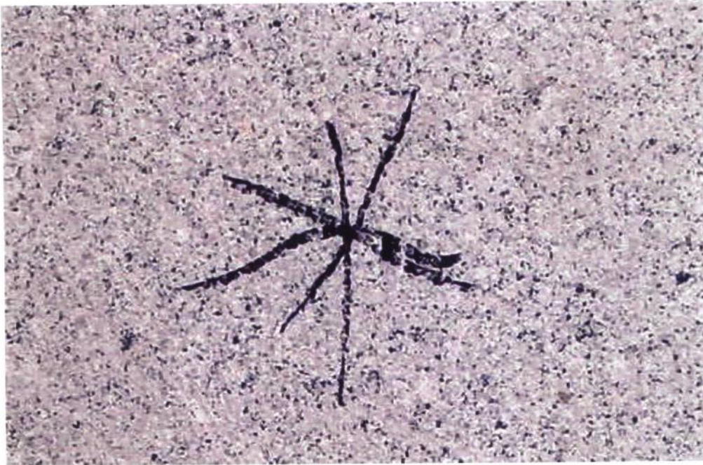
29. Surface with applied graffiti.
